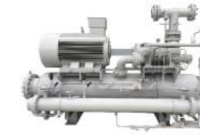
AMMONIA REFRIGERATION UNIT
